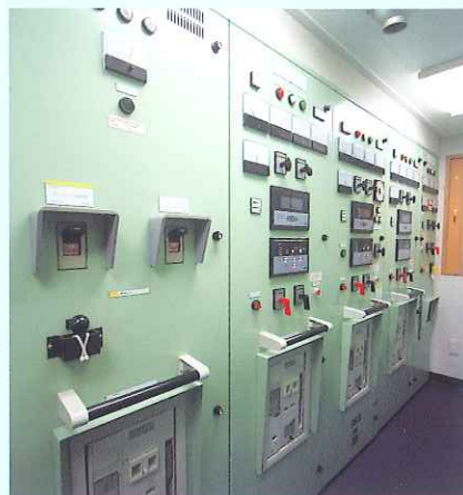
配電盤 / Switch board
