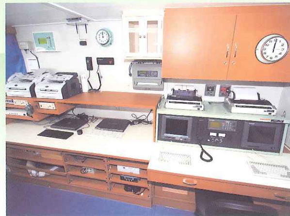
無線区画 / Radio equipment area
